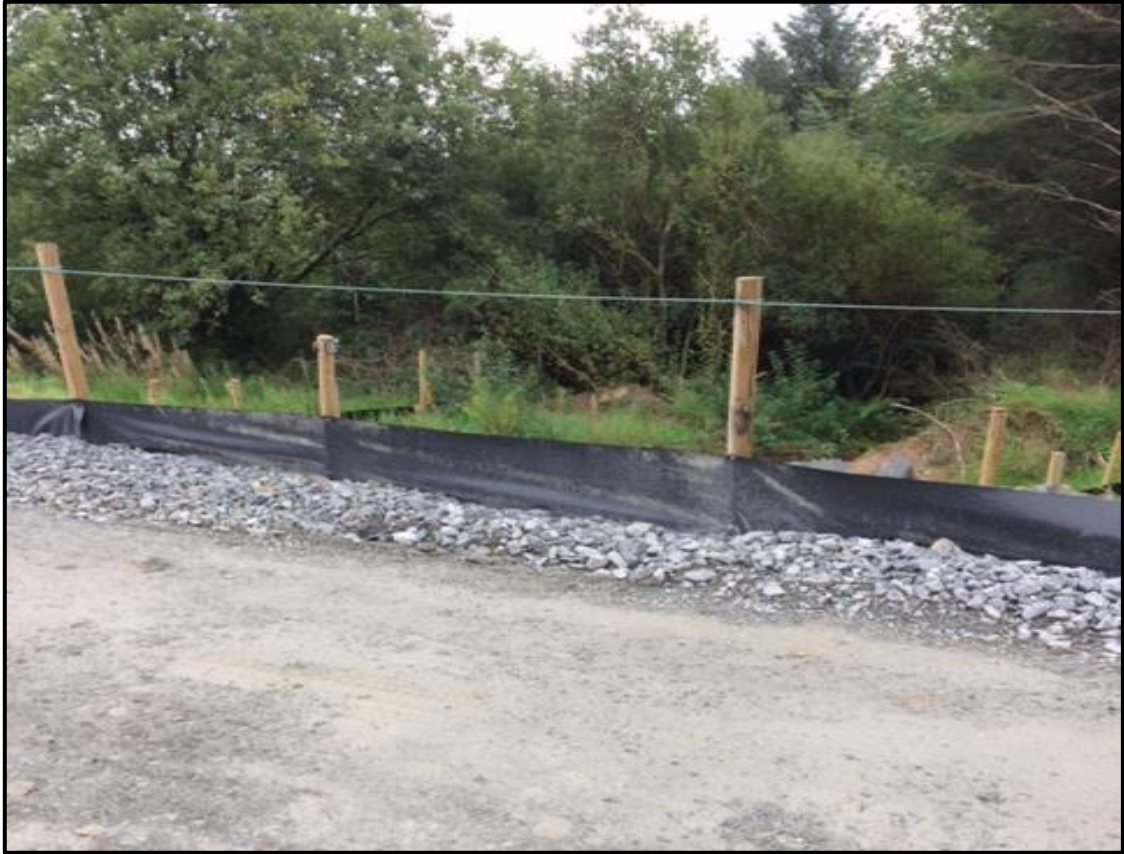
Figure 3-30 Dirty water containment at watercourse crossings
