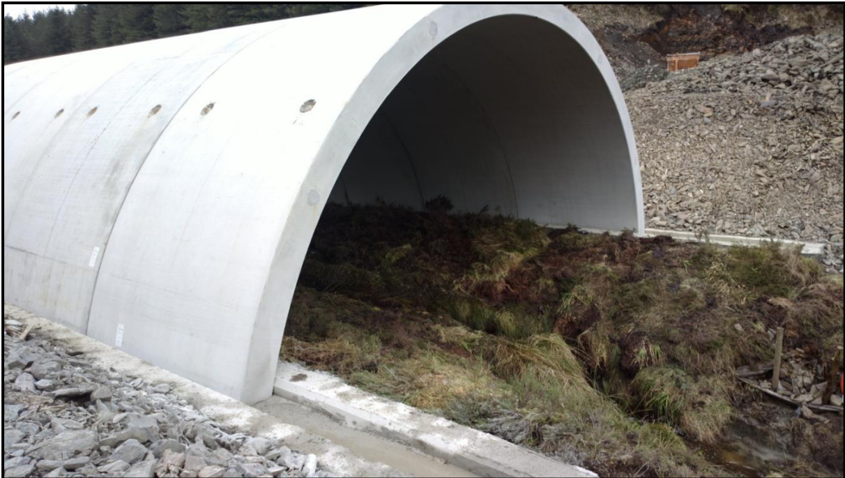
Figure 3-27 Typical clear span pre-cast concrete units in place over an existing watercourse
