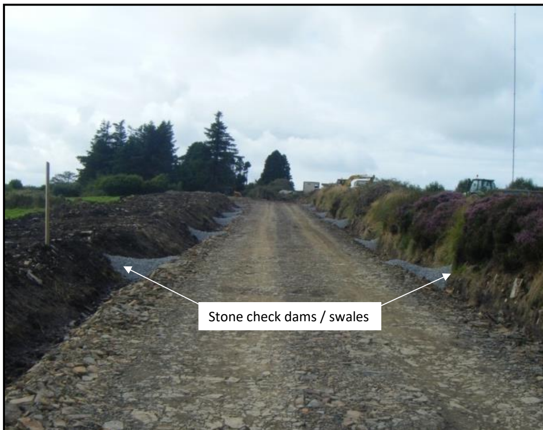
Figure 3-34 Examples of check dams along roadside drainage channels
