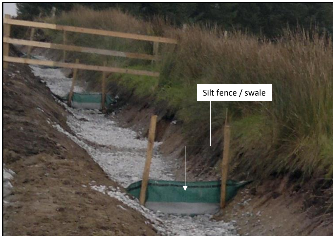
Figure 3-35 Example of a silt fence used in conjunction with check dams along roadside drainage channels
