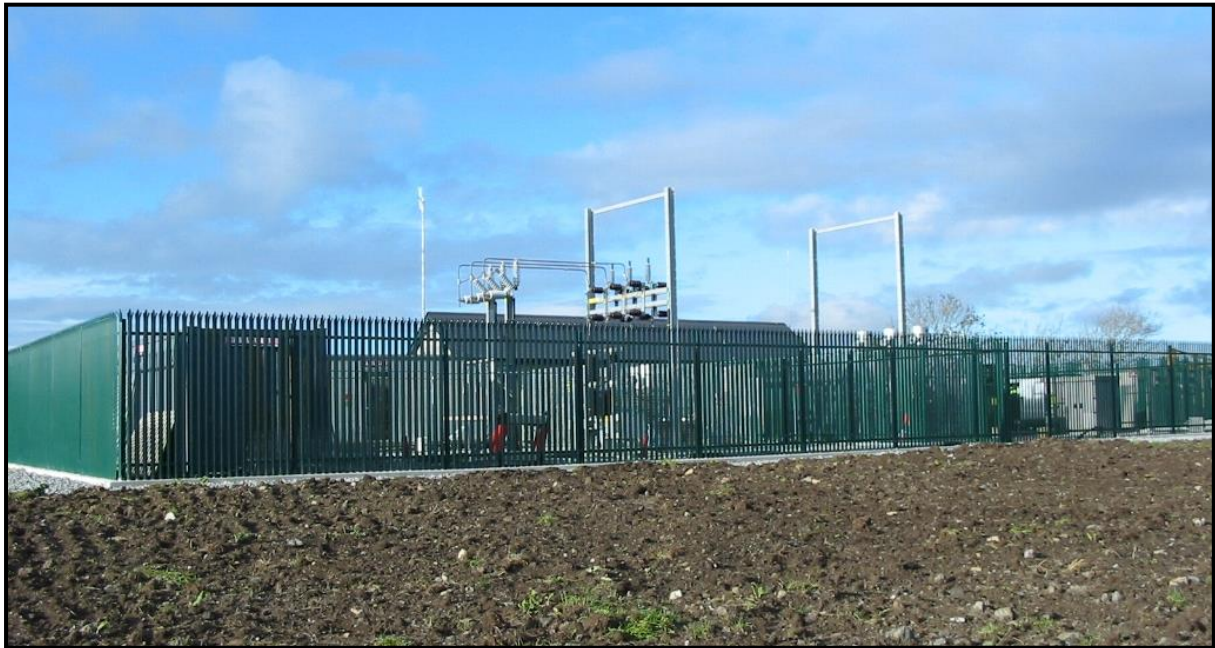
Figure 3-22 Typical substation building and compound
