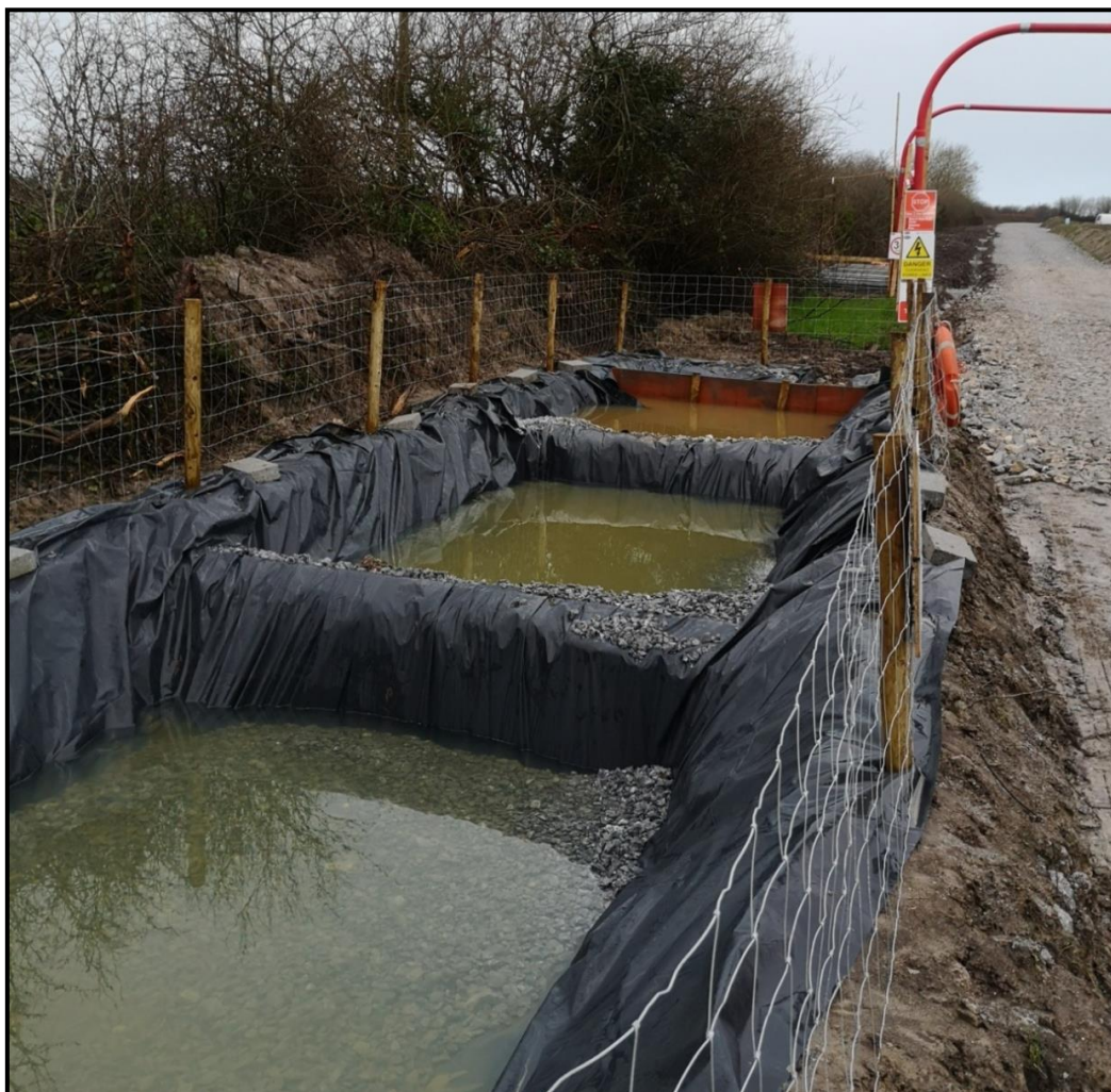
Figure 3-33 Multi-tiered settlement pond with stone filter
